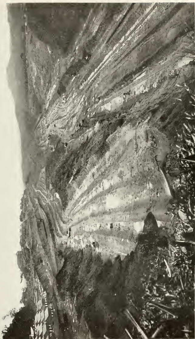
CULEBRA CUT, LOOKING NORTH FROM CONTRACTORS' HILL AND SHOWING TERRACES LEFT AFTER REMOVING SUPERIMPOSED WEIGHT TO AVOID "SLIDES."
